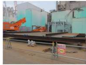
• Unit 4 Spent Fuel Pool protection platform Photo taken by a TEPCO employee on June 7, 2012
